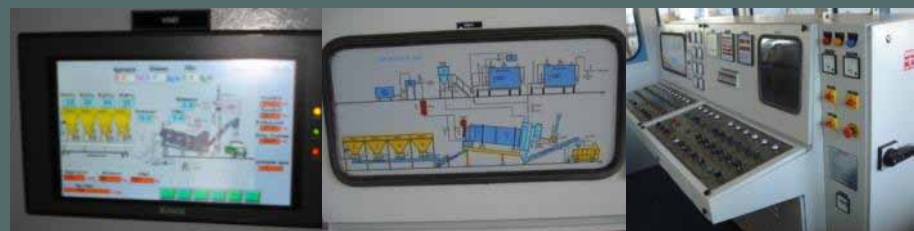
*** PLC TOUCH SCREEN TYPE PANEL
